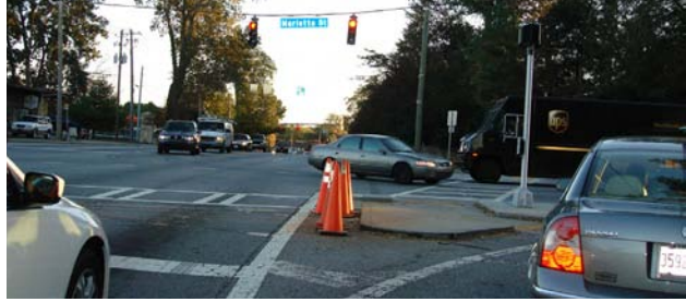
Hazardous pedestrian conditions at intersection of Atlanta Street and Marietta Highway.
