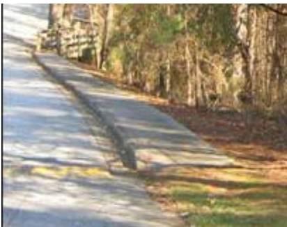
Hazardous surfaces, lack of curbs and buffers, and “sidewalks to nowhere” are common conditions for pedestrians.
